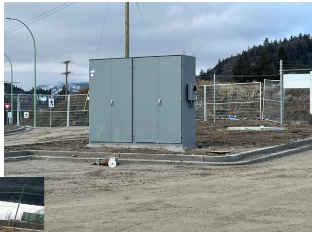
Electrical kiosk installed
