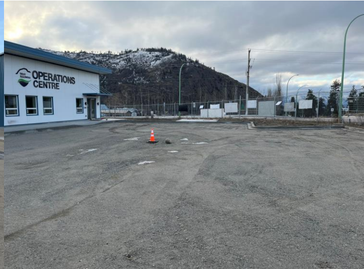
Grading and sub-base complete for Admin parking lot, berm removed, fencing installed
