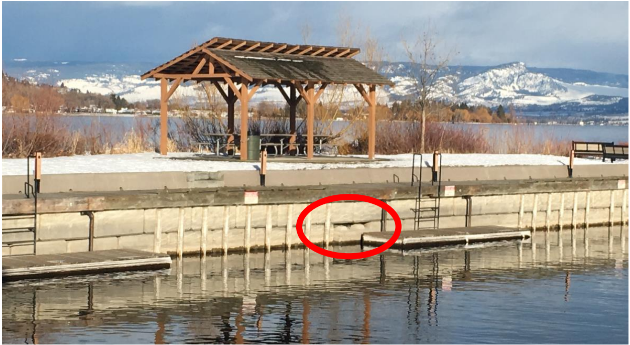
Photo 17: Project 46 – Gellatly Boat Launch - displaced lock block
