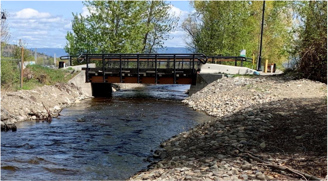
Photo 11: Project 19 – Lower Powers Creek – Gellatly Bridge w/ ~1m additional clearance under decking
