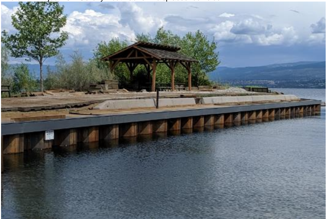
Photo 18: Project 46 – Gellatly Boat Launch – most cost effective repair was to retain lock block wall with sheet piles.
