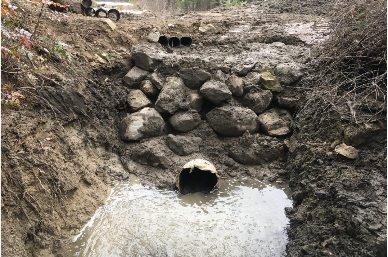
Photo 14: Project 13/26 – Rock Ridge Park – Culvert clean under sewer line and access road
