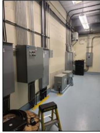
1 PHOTO 1 – MAIN ELECTRICAL ROOM E4 NTS
