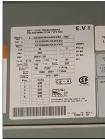
3 PHOTO 1 – 30 KVA TRANSFORMER E4 NTS
