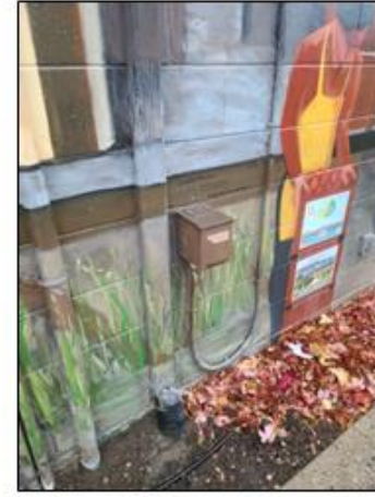
2 PHOTO 2 - ENERGIZED OUTLET (MUSEUM) E3 NTS
