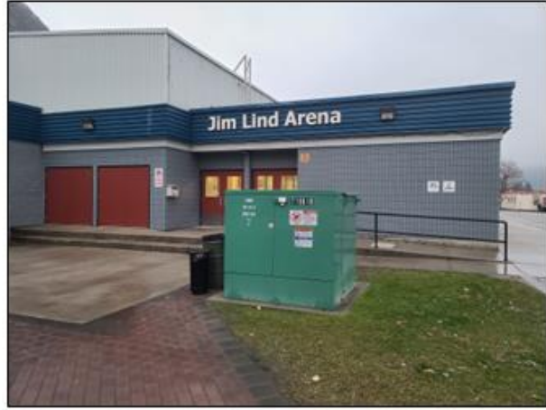
1 PHOTO 1 – PAD MOUNTED TRANSFORMER E4 NTS
