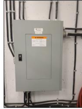
2 PHOTO 2 – SUB PANEL E4 NTS
