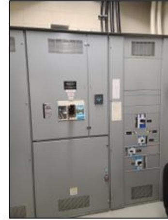
2 PHOTO 2 – MAIN SWITCHBOARD E4 NTS
