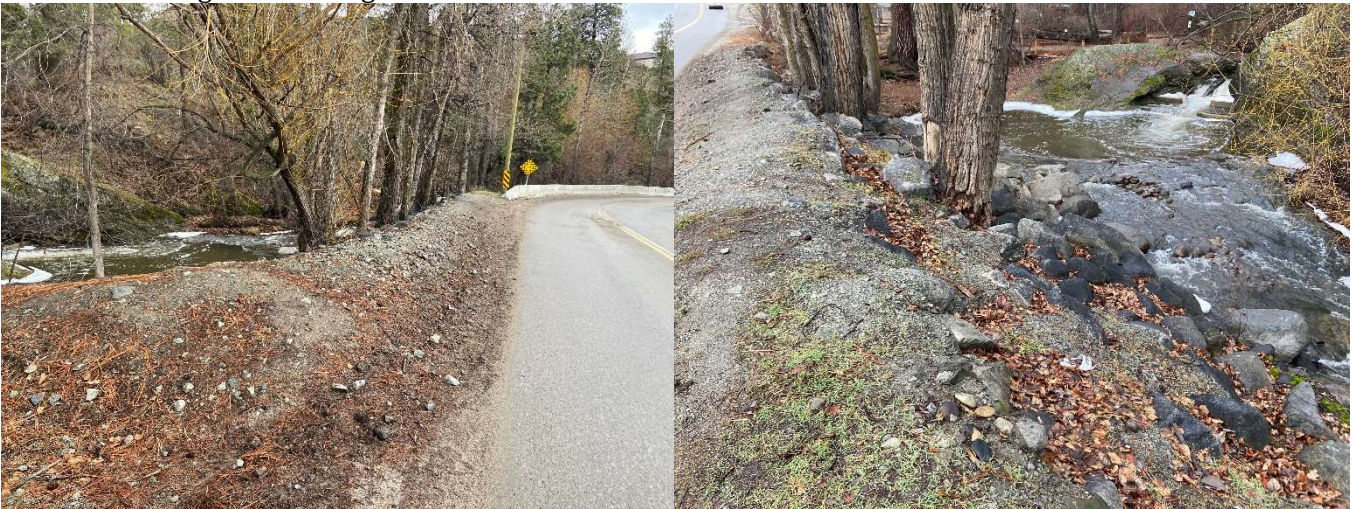
Figure 2 - Powers Creek Flood Protection along Right Bank at Glen Canyon Regional Park along Gellatly Road. Photos taken Jan 30, 2024. Looking downstream (left photo) and upstream (right photo)
