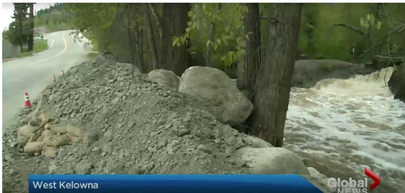
Figure 3 - Powers Creek emergency erosion protection at Glen Canyon Regional Park during 2017 flood event. Photo: GlobalNews.ca
