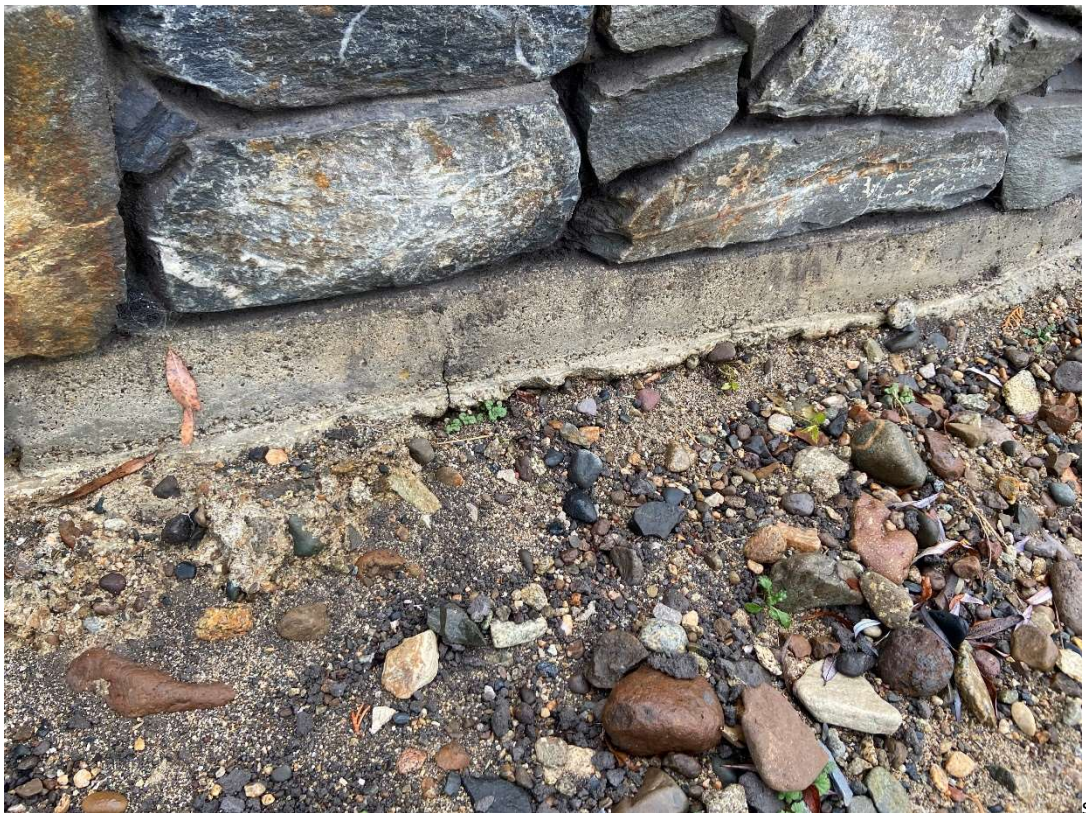
Photo 16: minor scouring under at lakefront retaining wall
