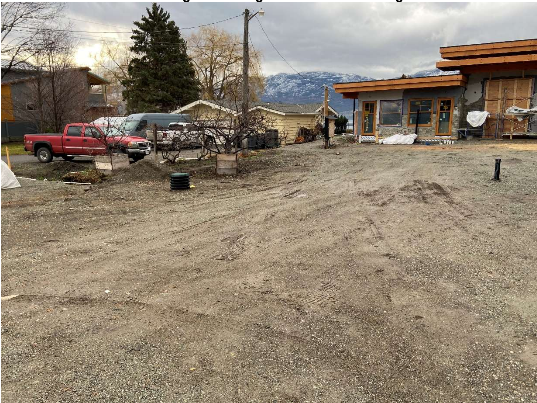
Photo 10: looking south at dwelling and rock pit (black HDPE Pipe in foreground)
