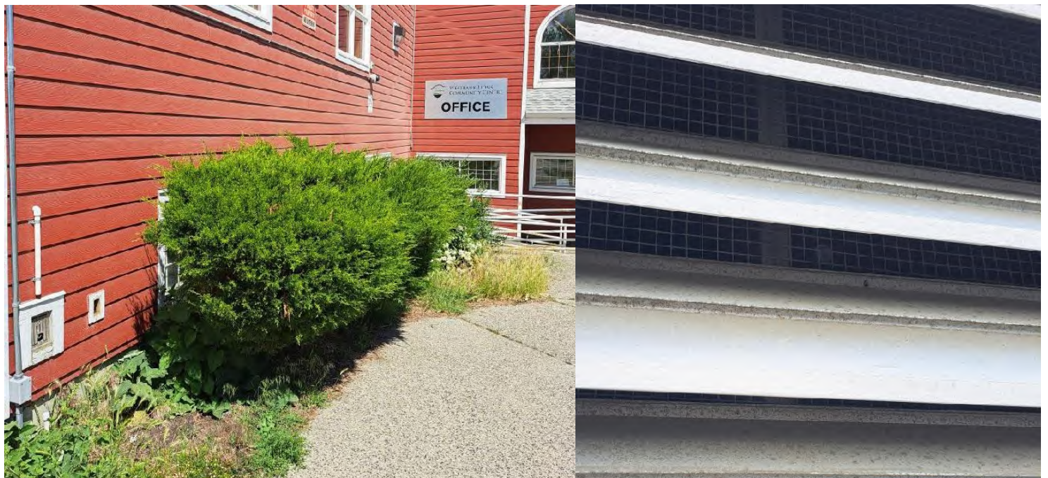
Figure 18. Common deficiencies noted during CI assessment, (left) flammable landscaping within Non-Combustible Zone of the Community Centre, (right) ventilation screening that is > 3 mm at the Johnson Bentley Memorial Aquatic Centre.
