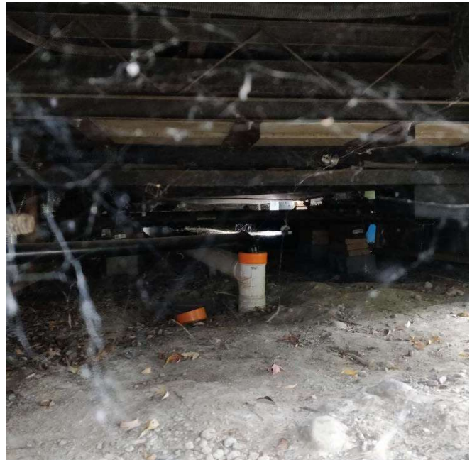
Figure 4 – View of Sanitary Connection under RV
