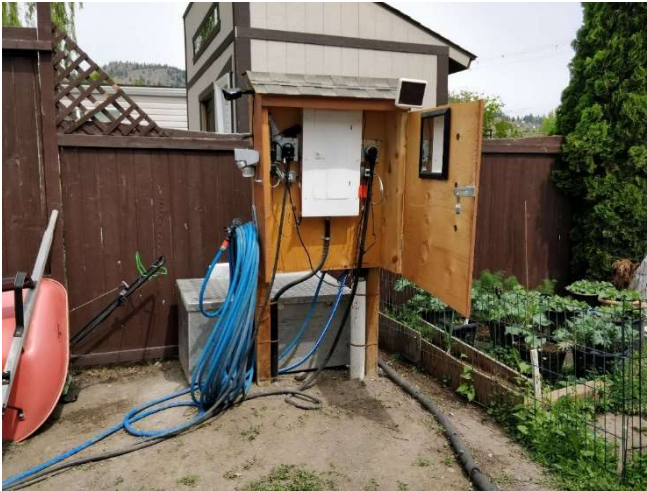
Figure 1 – Service Connections and Electrical Panel
