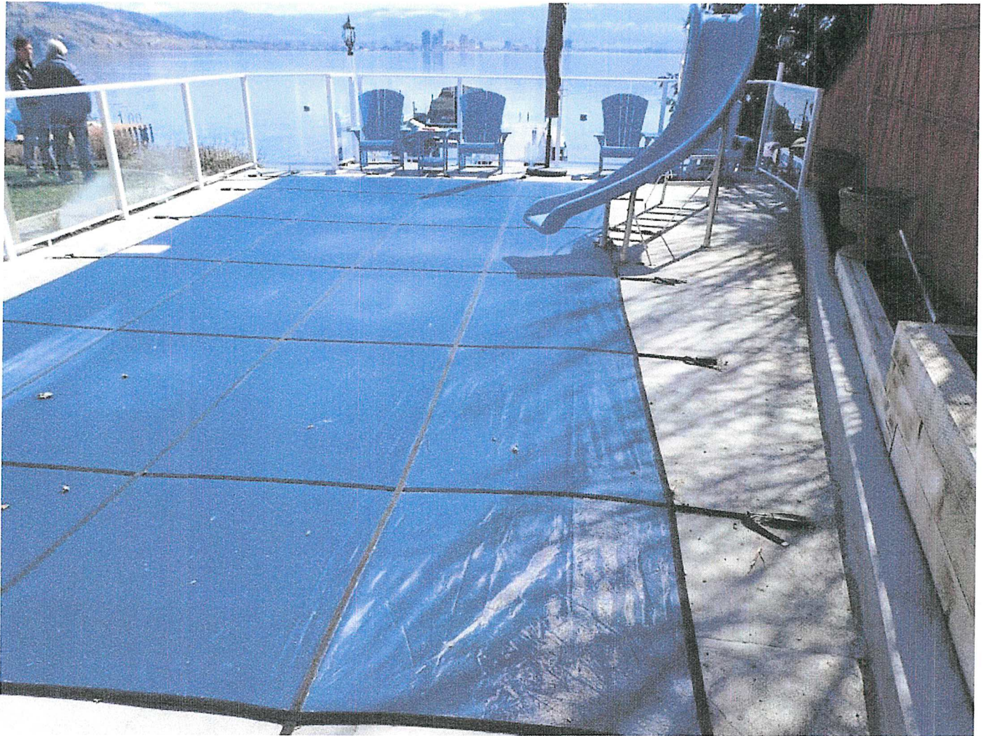
Photo 7. A view of the pool deck showing the current design. The proposal is to realign the pool with the property edge on the right and extend the pool area to the forefront. The wooden retainer along the right of the photo will be replaced with a rock gabion structure which will support the edge of the new pool.
