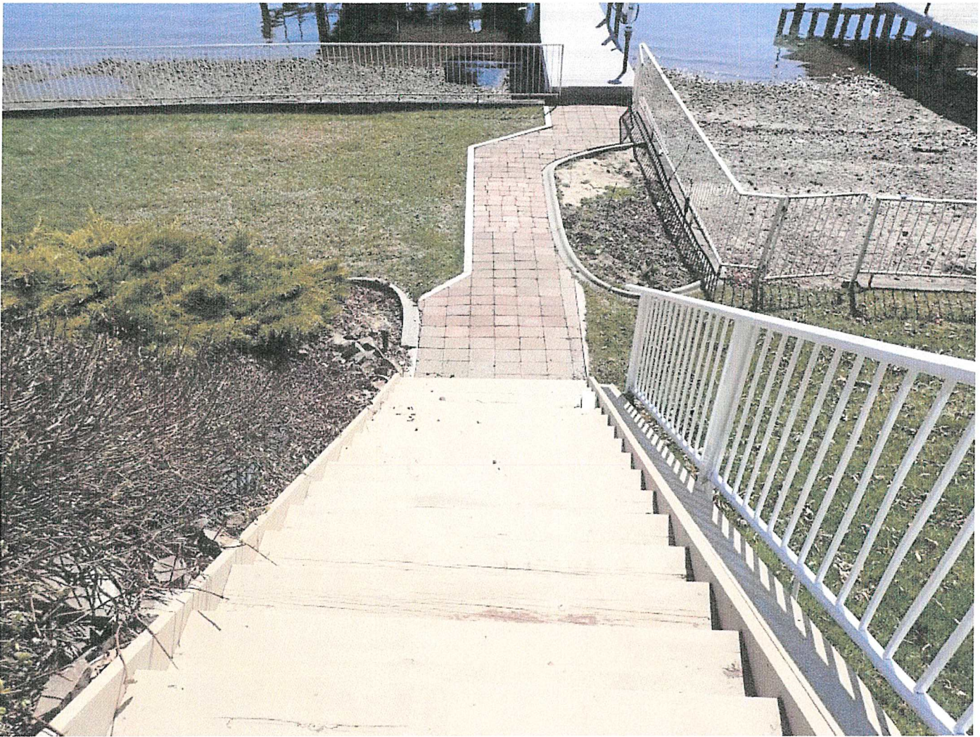
Photo 8. A view of the wooden staircase which connects the upper pool deck to the lower dock level. The proposal calls for a redesign of the wooden staircase which will be replaced with concrete slab steps placed into the bank and shifted slightly to the left of the existing steps in the photo. The tile connecting the pool will also be replaced with a new tile design. The grass area to the right of the railing will be replanted with native vegetation consisting of shrubs.
